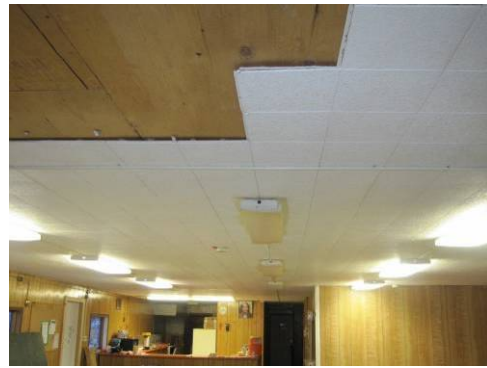
Missing Ceiling Tiles and Lighting System
