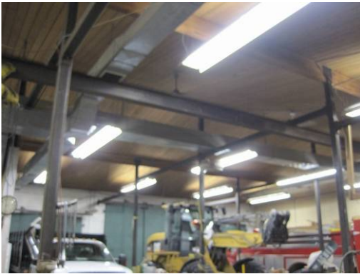
Garage Lighting System
