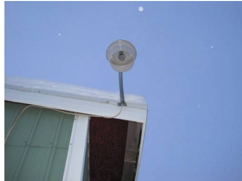
Exterior Lighting Fixture
