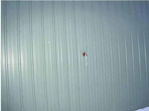
Minor Damage to Exterior Façade
