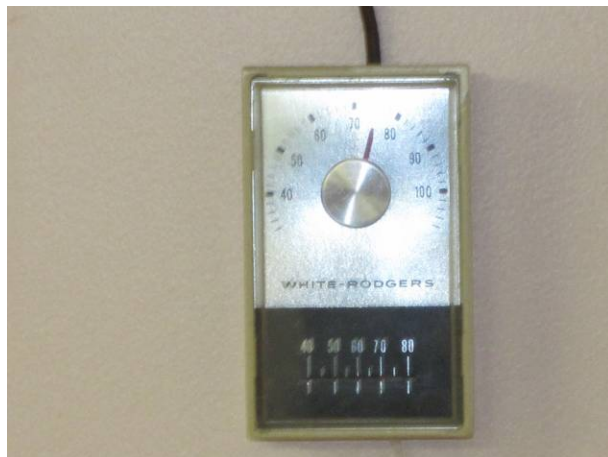
Thermostat for Entire Building
