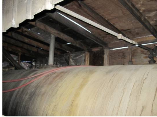
Gaps in Structure to Outside Conditions
