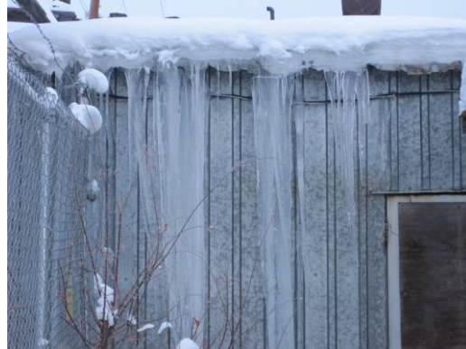
Ice Melting From Generator Heat
