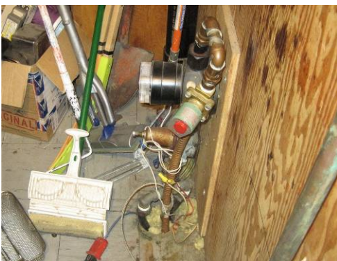
Poorly Insulated Penetration
