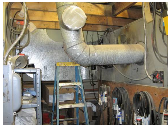
Heating System in Garage
